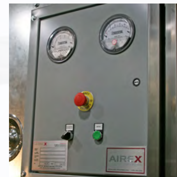
Inside Emergency Button
